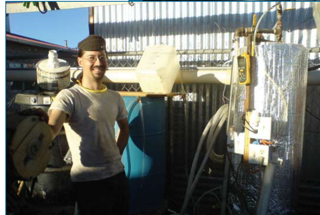
The refinery, a recycled hot water heater with insulation and attachments.
