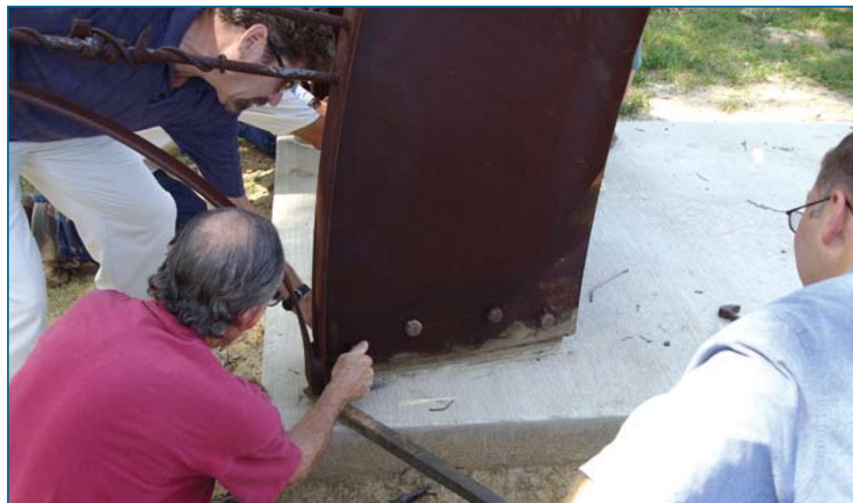
Bolting the bridge to the anchor system in the concrete foundation on the bank of the Mississippi River in Memphis.
